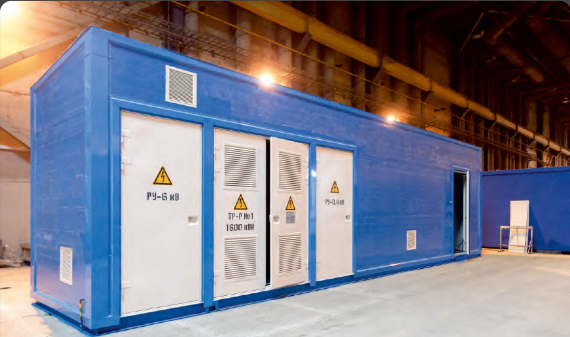
The Sredne-Nevisky Shipbuilding Plant Packaged Transformer Substation (PTS) 10/0,4 kV 1600 kVA
